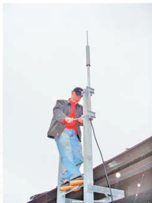
Frank Correia of Cape Ferrelo installs the antenna. Frank also fabricated the brackets, made with materials donated by Tom Blanchard of Brookings.
